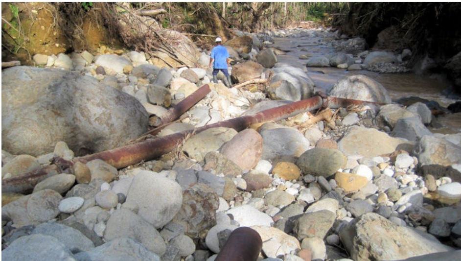
Photo 1. An old water distribution pipe that was damaged during Hurricane Maria lies on a river bed in Dominica. Photo courtesy of Marcel Misuraca (OCWA)
